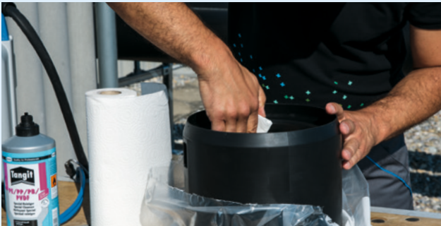
Clean the fusion zones of the fitting and pipe using a clean cloth.
