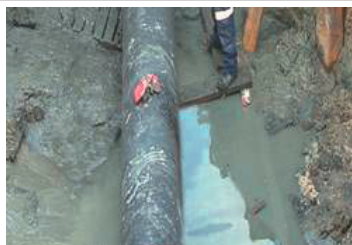
Water residues must be pumped off
